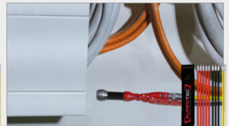
Shafts and underfloor ducting
